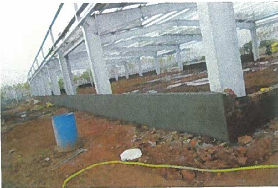
PEB factory structure at Chhindwada Call Centre: The brick wall constructed in long line structure since there is no direct load at the moment on the structure; it remains to be seen how the brick wall behaves under the stress of weather and vertical cladding as single line wall.
